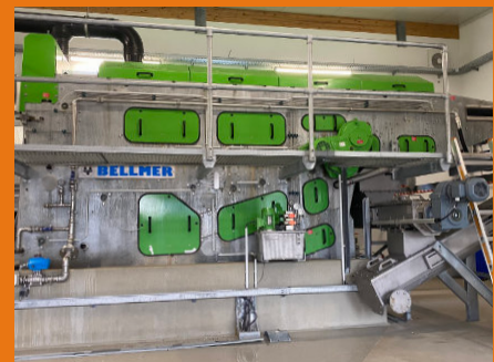
Lubrication system on belt press
