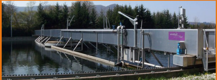
GMF pump in operation on the circular scraper
