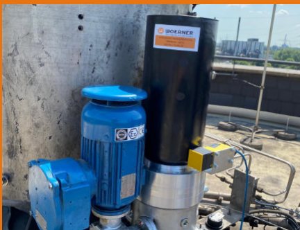
ATEX Kx cartridge on the digestion tower
