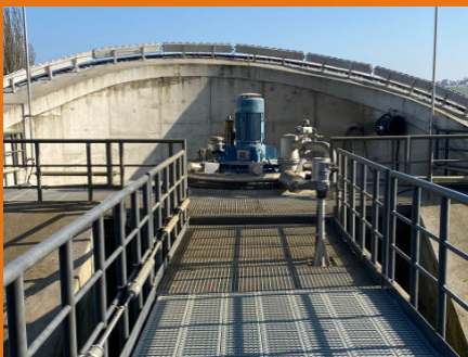
GMF on various digestion towers
