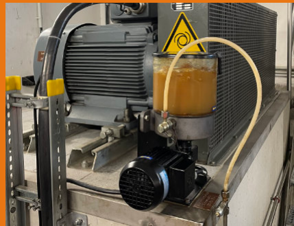
In the pump house: GMA for bearing lubrication on the screw drive
