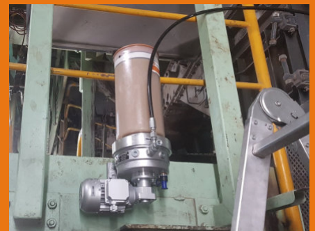
Central lubrication pump with Kx for bearing lubrication
